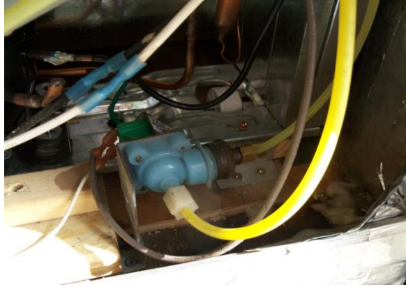
Water Valve & Leveling Block
