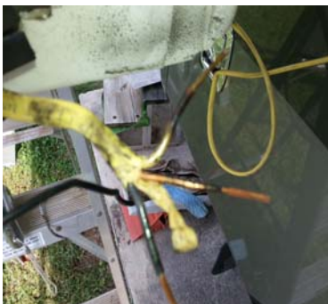
Photo 5: A close-up view of the burnt wires.
