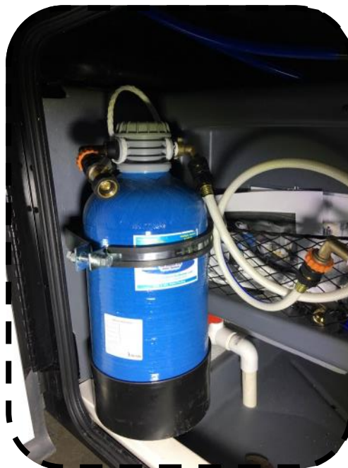
Water Softener is installed
